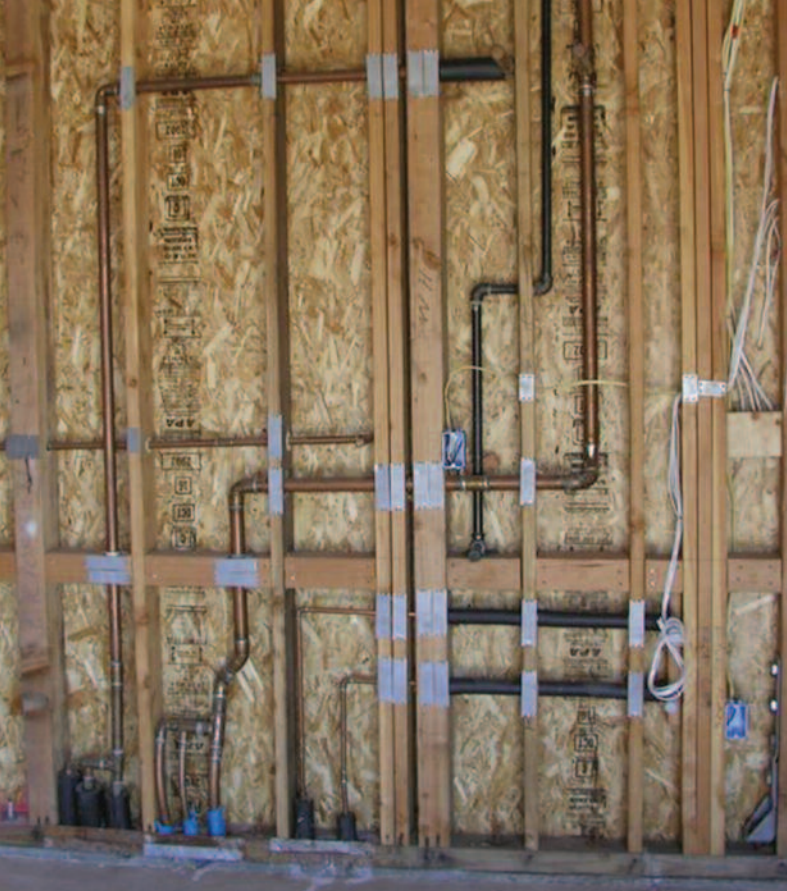
Hot and cold potable supply piping (left) and 1/2 inch return lines (center) for a slab-on-grade house.
