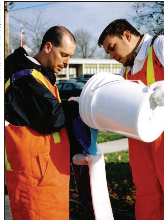
Trenchless technology installers pour resin into a liner that will be positioned into place inside the damaged area of the pipe.
